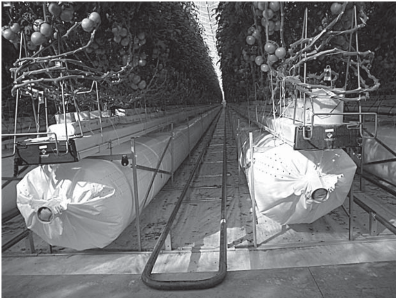
FIGURE 10.59 FormFlex gutters as raised trays above the convection tube. (From Eurofresh Farms, Wilcox, AZ. With permission.)
