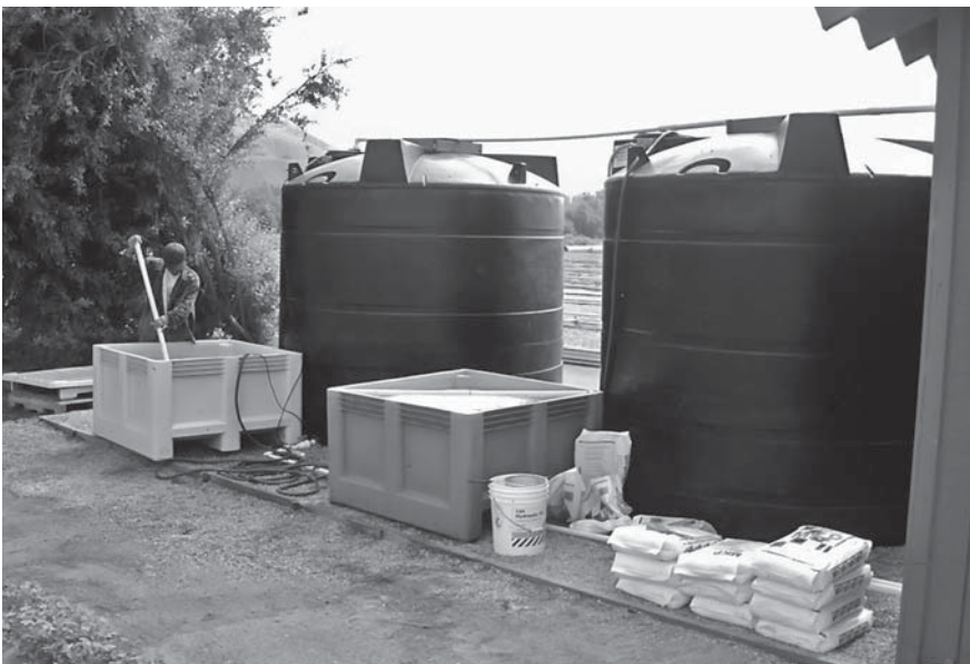
FIGURE 3.9 Image of 2,300-gal stock tanks with injector shed. (From California Watercress, Inc., Fillmore, CA. With permission.)
