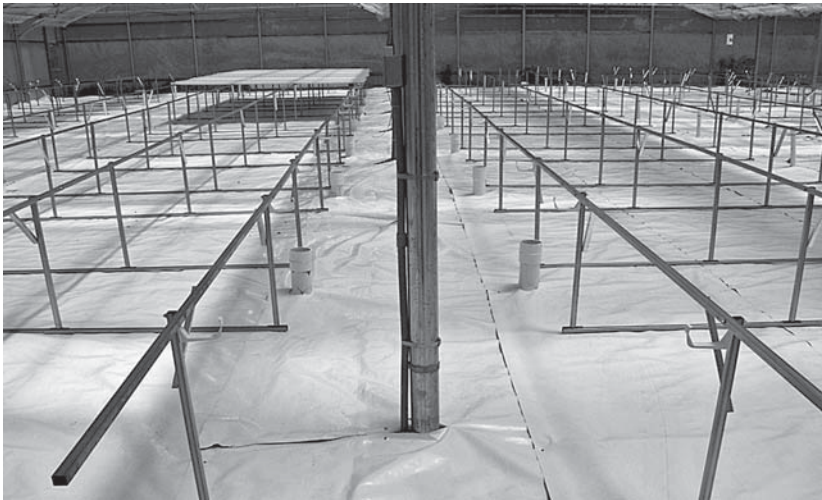
FIGURE 6.4 Benching system constructed for support of the NFT channels. Note: The channels placed on the bench in the back. Also, note that the benches are sloping toward the greenhouse side-wall posts and there are 3-in. PVC drain pipe risers for the catchment trench to drain to for return to the nutrient cistern. (From American Hydroponics, Arcata, CA. With permission.)
