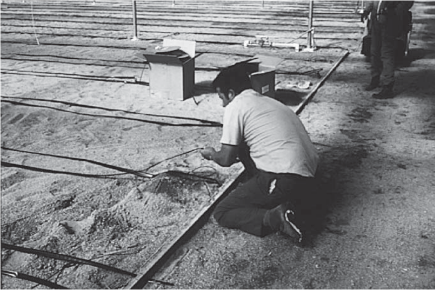
FIGURE 8.5 The installation of ooze hoses for an automated drip irrigation feeding system.
