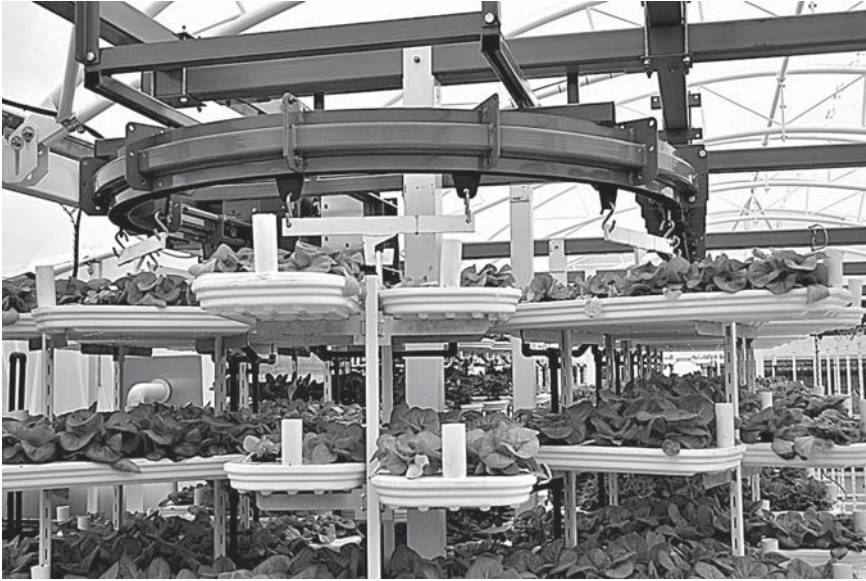
FIGURE 13.44 The drain lines at the back of the trays. (From Valcent Products [EU] Ltd., Cornwall, UK. With permission.)
