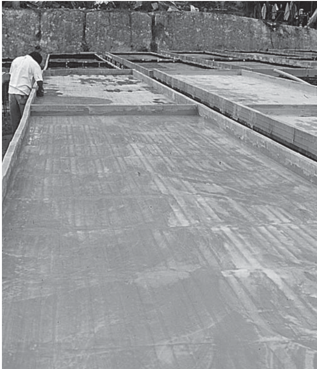
FIGURE 13.6 Beds leveled with a coat of concrete. (From Hidroponias Venezolanas, S.A., Caracas, Venezuela. With permission.)
