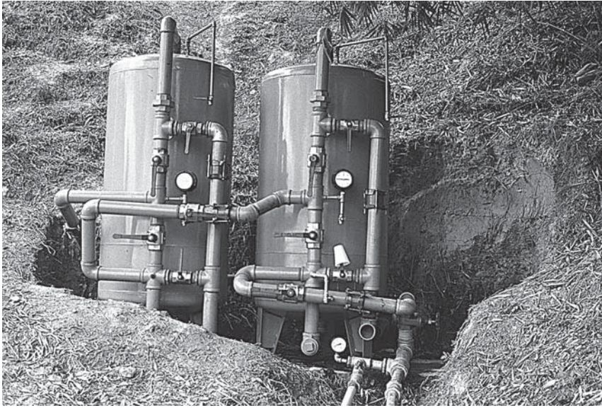
FIGURE 13.1 Filtration system of mountain spring water source. (From Hidroponias Venezolanas, S.A., Caracas, Venezuela. With permission.)
