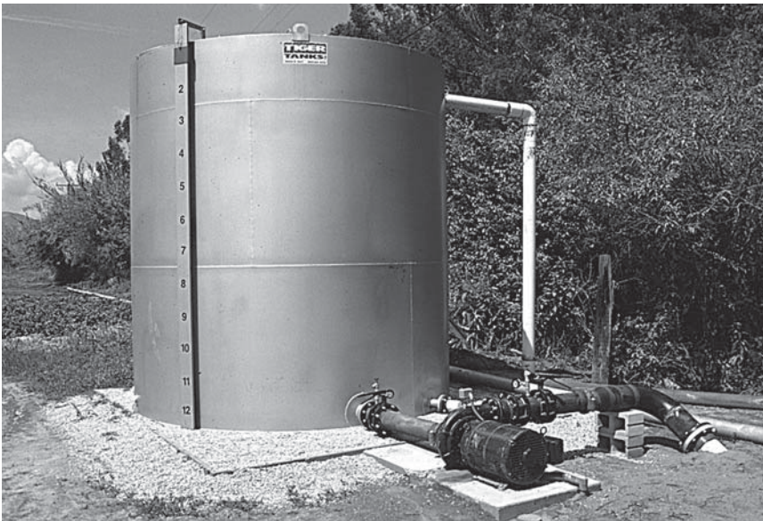
FIGURE 6.55 Booster pump pressurizes 8-in. main water line from 10,000-gal tank, which is filled from a well. (From California Watercress, Inc., Fillmore, CA. With permission.)
