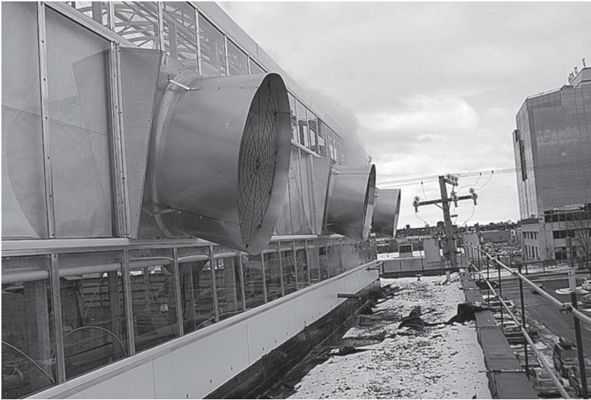
FIGURE 13.33 Exhaust fans on the side opposite to the cooling pad. (From Lufa Farms, Montreal, Canada. With permission.)
