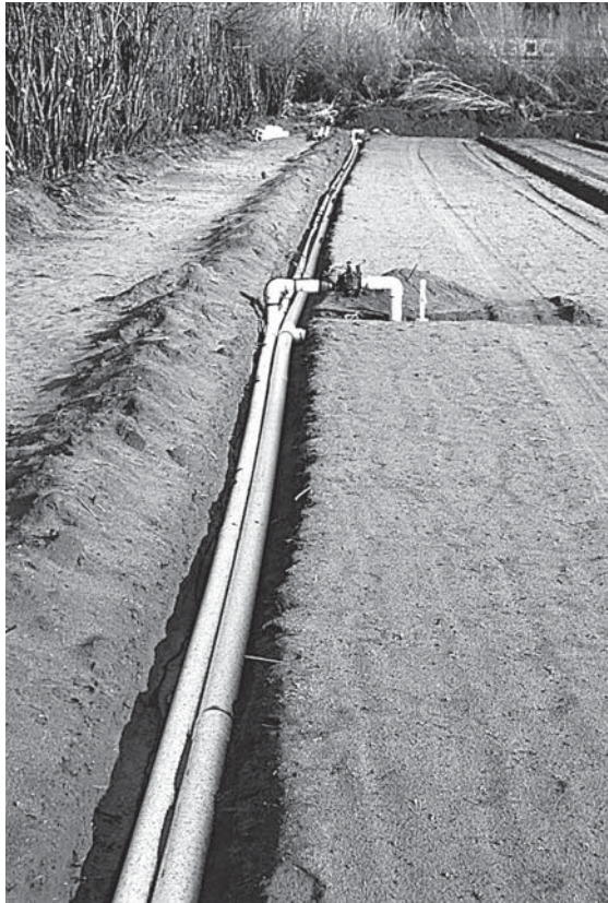
FIGURE 6.49 Irrigation mains at side of field. Four-inch-diameter raw water main and 3-in. nutrient solution main. Note: Risers to solenoid valves of 2-in. submains going across the field. (From California Watercress, Inc., Fillmore, CA. With permission.)
