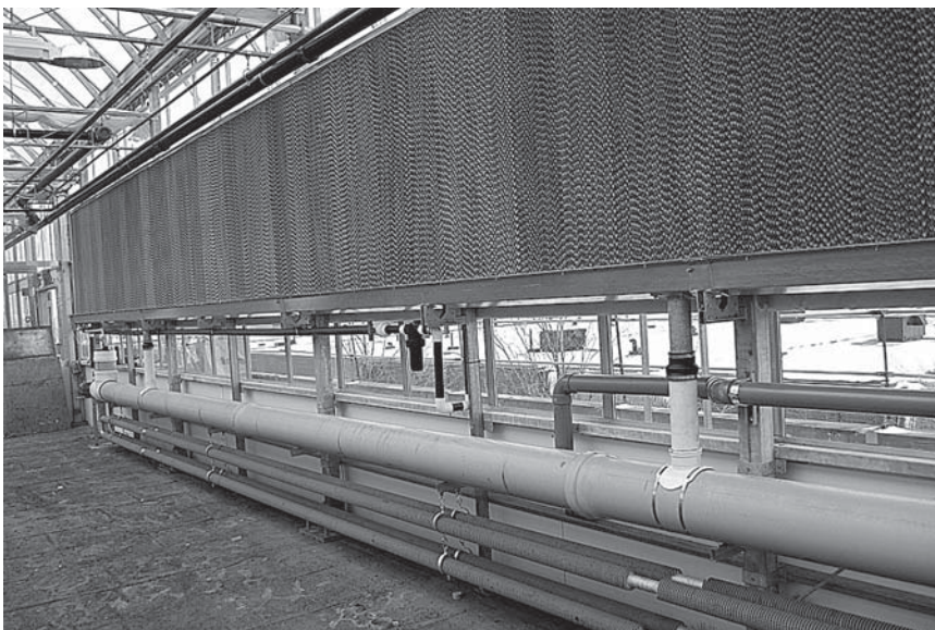
FIGURE 13.32 Evaporative cooling pad. (From Lufa Farms, Montreal, Canada. With permission.)
