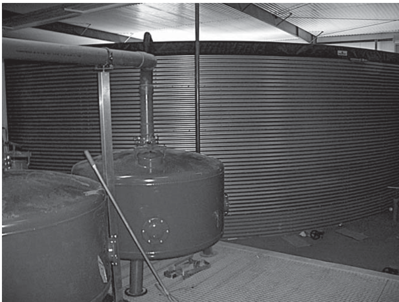
FIGURE 10.61 Sand filters with return tank. (From Eurofresh Farms, Wilcox, AZ. With permission.)
