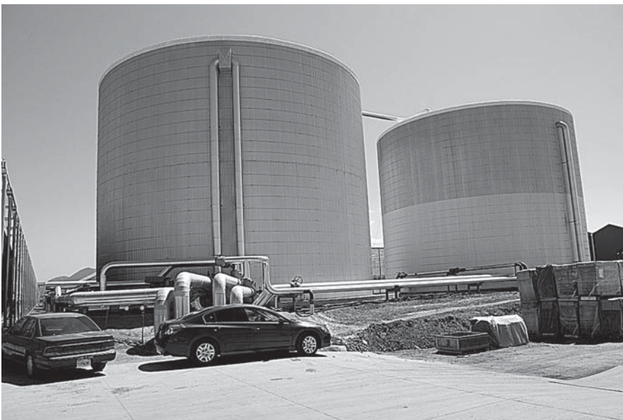
FIGURE 11.14 Hot water storage tanks. (From Houweling Nurseries Oxnard, Inc., Camarillo, CA. With permission.)
