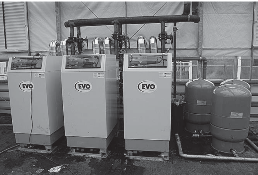
FIGURE 13.34 Hot water boilers for heating system. (From Lufa Farms, Montreal, Canada. With permission.)
