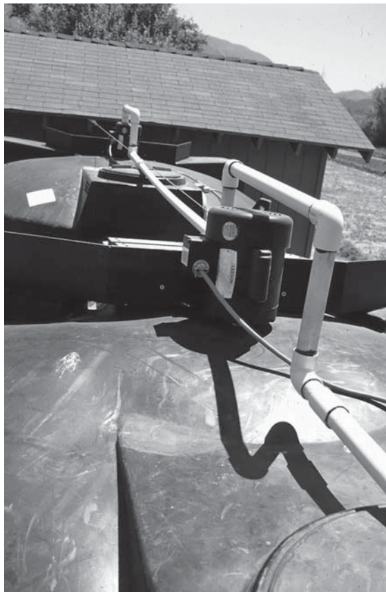
FIGURE 3.7 Stock tanks (2,300 gal) A and B with circulation pumps. (From California Watercress, Inc., Fillmore, CA. With permission.)
