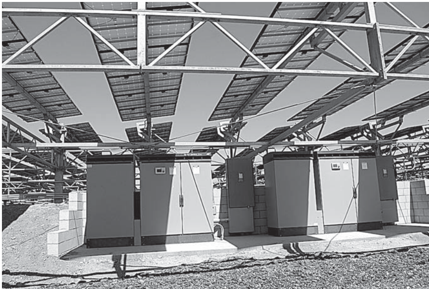
FIGURE 11.8 Tilting solar panels above electrical panels. (From Houweling Nurseries Oxnard, Inc., Camarillo, CA. With permission.)
