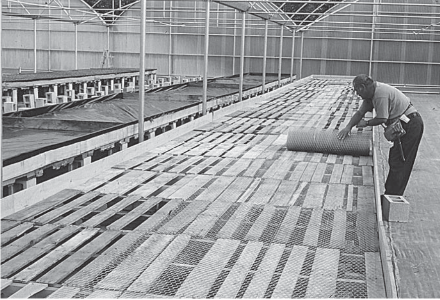
FIGURE 12.2 Beds are lined with chicken wire to support a polyethylene liner. (From California Watercress, Inc., Fillmore, CA. With permission.)
