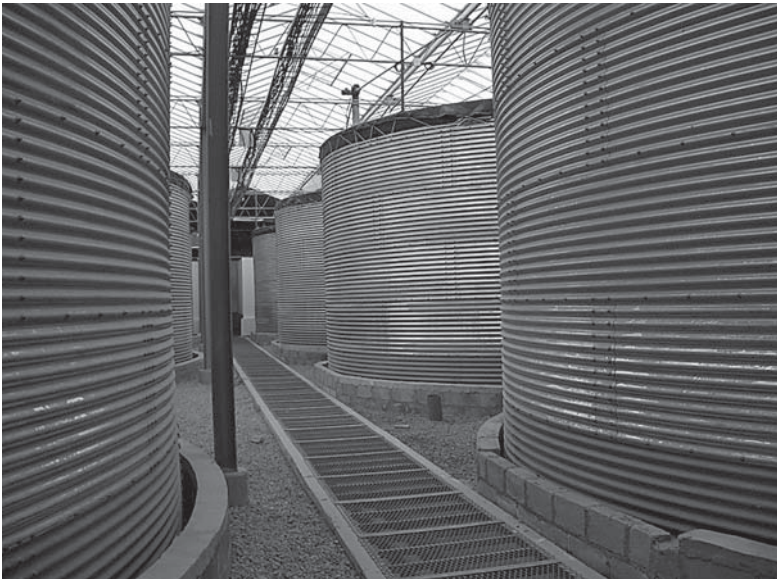
FIGURE 3.11 Large nutrient solution collection tanks in a closed system. (From Bionatur Invernaderos Biologicos De Mexico, S.A. De C.V., Jocotitlan, Mexico. With permission.)
